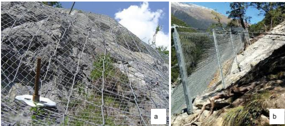
Figure 1 : Steel net protective element (a) fixed on the bedrock by nails and (b) located at the base of the bedrock
